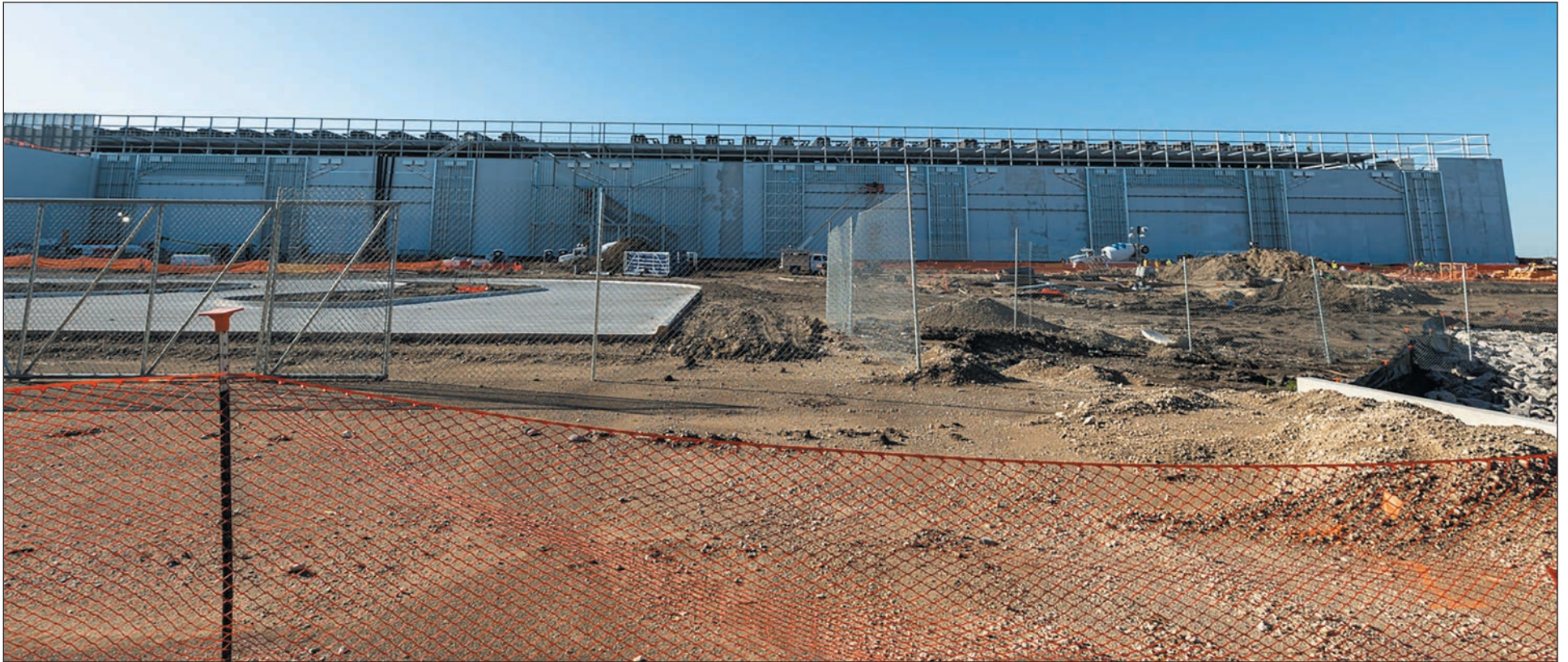
This data center in Wilmer, TX, is currently under construction. Opponents of the proposed Project Jupiter Data Center in Doña Ana County, NM, gained a victory against the project recently, which had to scrap its plans to power the center using a huge methane gas plant. Despite retracting their request for an air pollution permit amounting to more than NM's three largest cities — Project Jupiter is back with a new proposal to use methane gas fuel cells. Comments on this new proposal are due on July 6th. Visit riograndesierraclub.org to make a comment before the deadline. Photograph courtesy of Rick Baraff.
